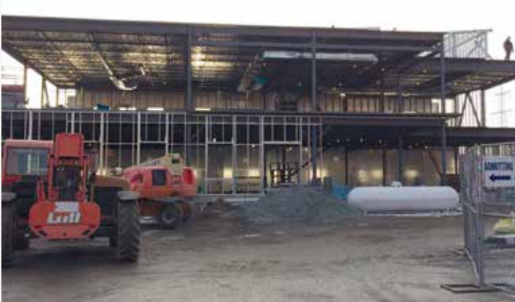
A look inside the front entrance of the new Animal Center in late December.
